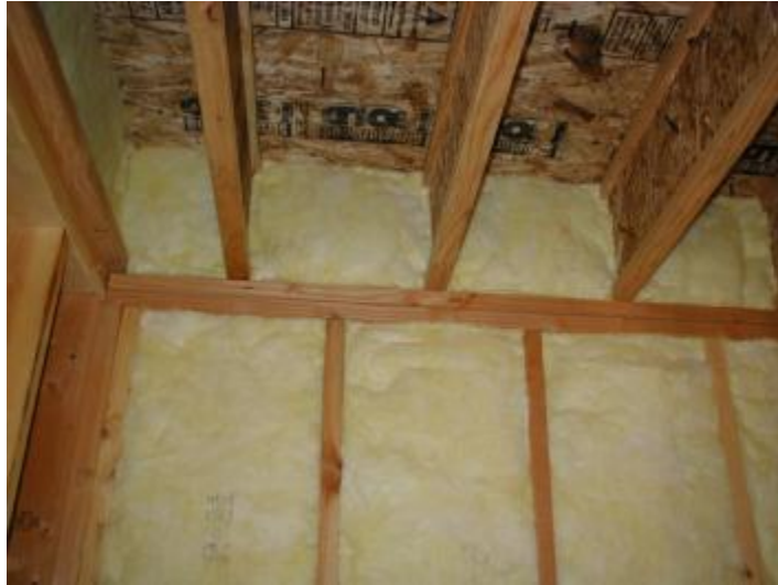
Figure 2: Example of Quality Installation of High Density Fiberglass Batt
