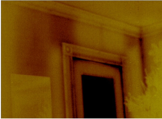
Image 4. Properly installed cellulose is an excellent insulation. Unfortunately it is often poorly installed with missed areas and settling the most common quality problems.
