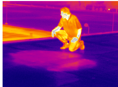
Image 10. The wet insulation in the roof system shows up clearly due to its greater thermal capacitance.
